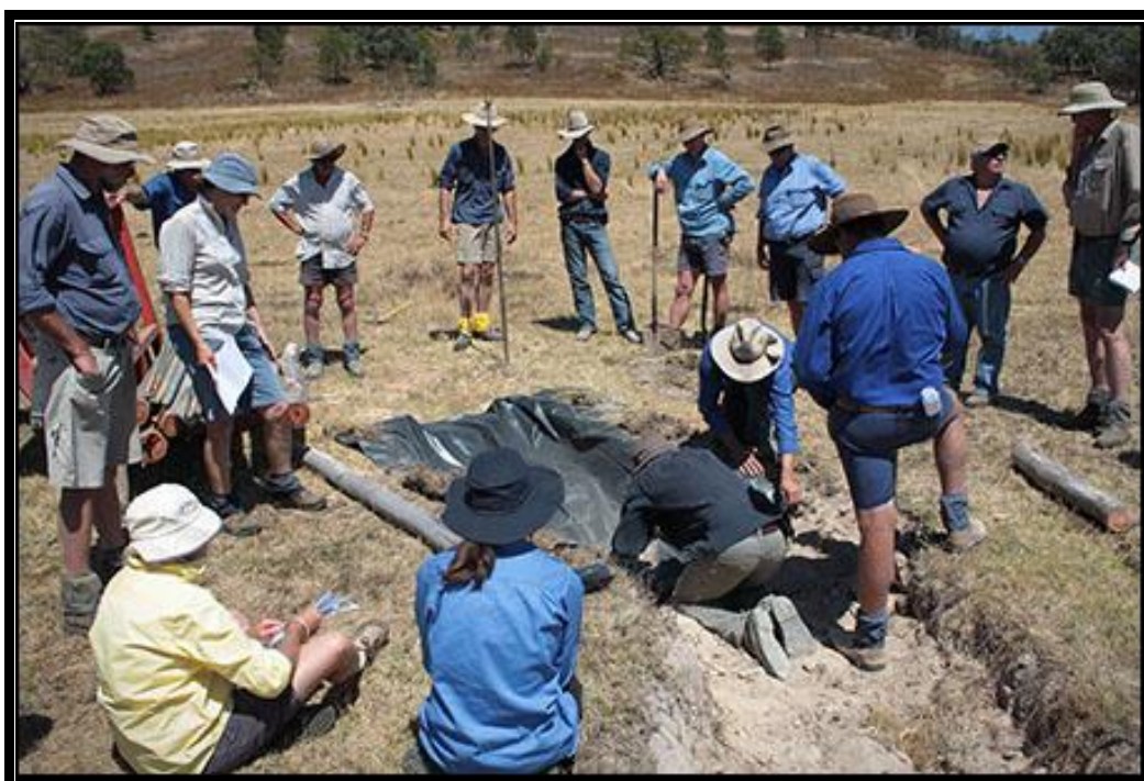
Above: Lining a gully-head with plastic to reduce dispersion of sodic soil, 2012.
